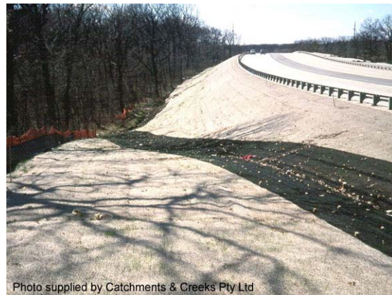
Photo 2 – Placement of erosion control blankets (beige) on road batter, with permanent erosion control mat (black)
